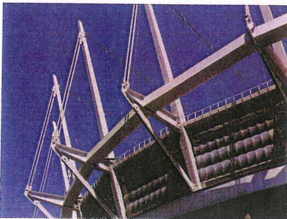
Figure 18.11 Single-layer ETFE film creates an effective clerestory below the new roof on Vancouver's BC Place Stadium.
